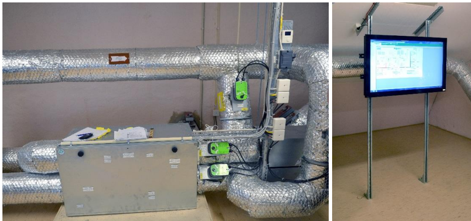
Figure 23. Picture of the ventilation unit; a Systemair VR 700 DC, and a monitoring screen located in the attic.
