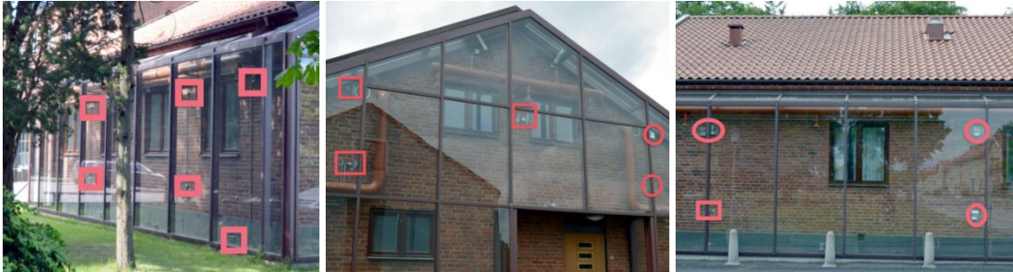
Figure 49. Sensors located on the west (left), south (middle) and east (right) facades. The unshielded sensors are marked by the red rectangles, and the shielded sensors by red circles.
