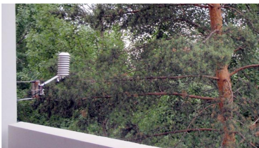
Figure 18. Outdoor weather sensor inside the factory-made outdoors sensor guard.
