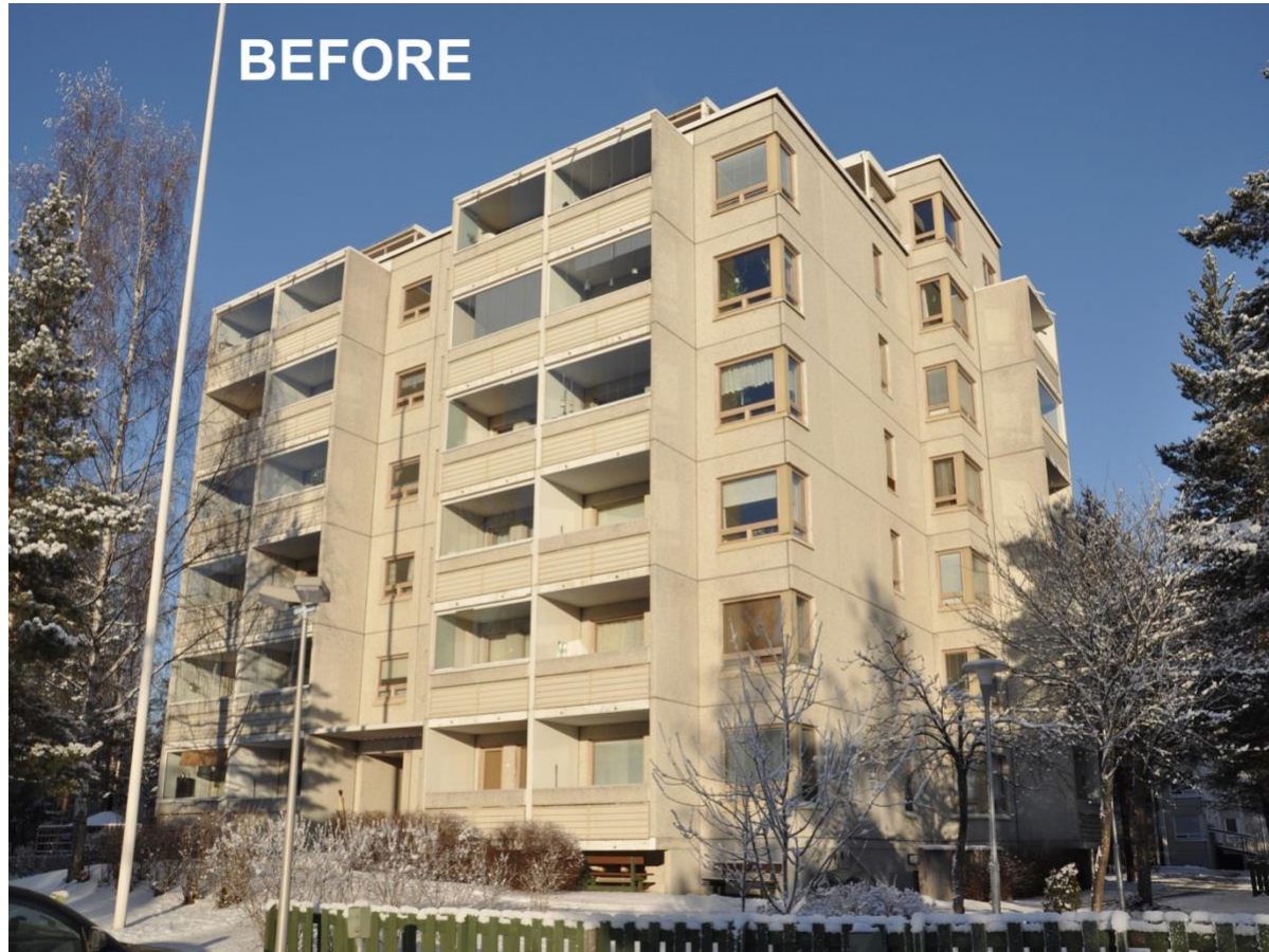
This existing multi-unit residential building has unenclosed balconies and is beginning to show signs of aging façade. It is a candidate for a comprehensive retrofit to address updating of its appearance and performance.
